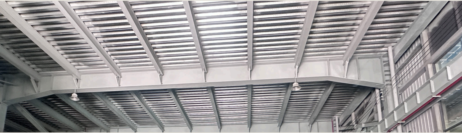
Roof interior / application reference
